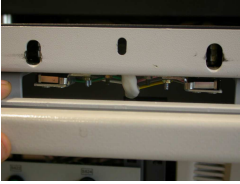
DSCN1001 is a picture of both lower switches
