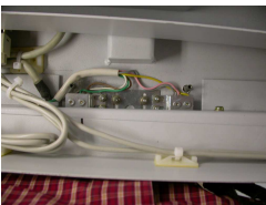
DSCN0997 is a picture looking down both upper switches with the cover removed
